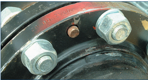
Figure 5. Close-up of the permanently attached pin on the facility vapour connection. Notice the insulating kit, the white insulating washers are visible.
