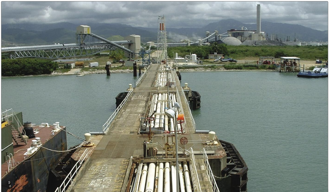
Figure 4. Loading Pier with the MVCS end control device, a Vapour Recovery Unit, shown at the end and to the right hand side of the pier.
